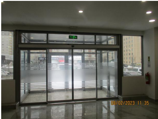
Fire Emergency Exit sliding door (NC).JPG
