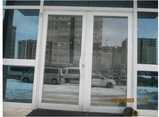
Fire Emergency Door opens inwards (NC).JPG
